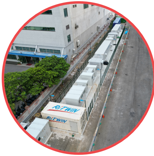
4MW/5.2MWh 鋰鐵電芯 (LFP)
